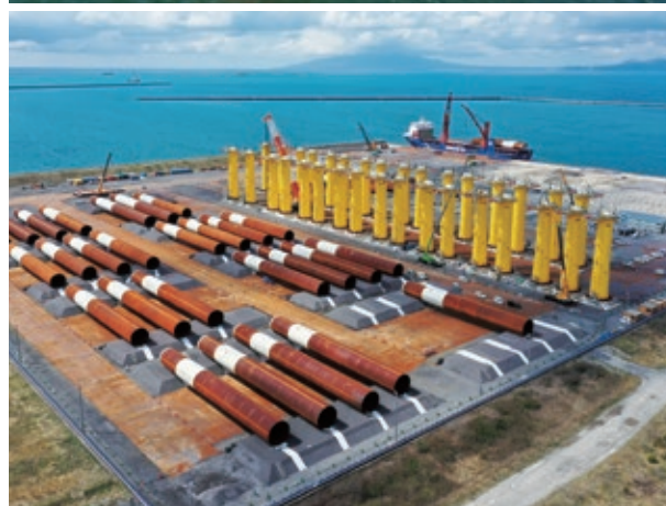
Akita Port & Noshiro Port Offshore Wind Farm Projects (Above) SEP vessel in operation (Below) Panoramic view of the pre-assembly yard for wind turbine foundations
