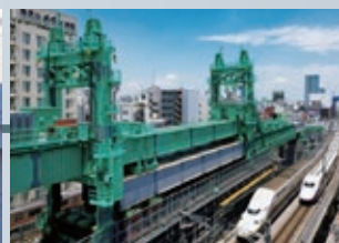
East Japan Railway Company Ueno-Tokyo Line
